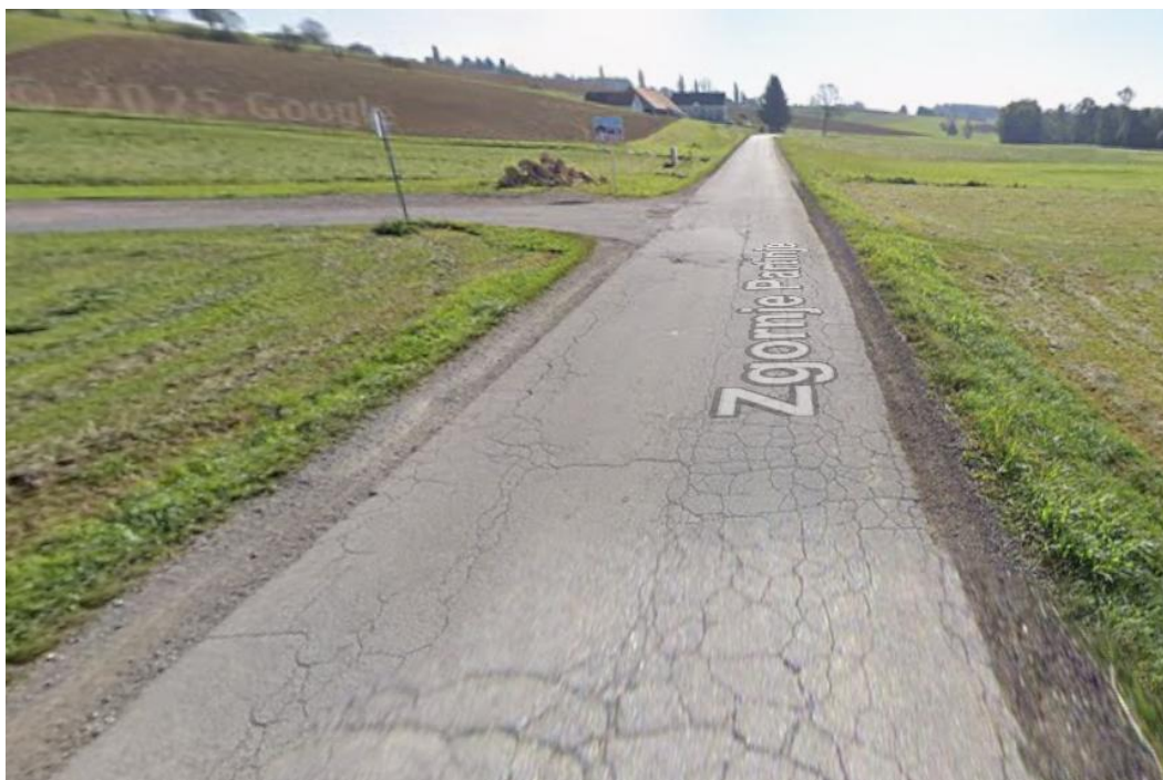
Slika 29: Dotrajana cesta LC 203 141 (vir: Google street view)
